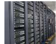
Data-Center SDN SAN Storage iNIC, vNIC T4/T2 PCIe Card
